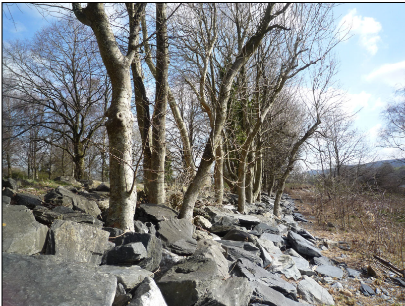
P3 – Base of trees in G1 growing out between gaps in existing embankment. Many boulders have become embedded in stems & there is insufficient space for further establishment without potential fractures
